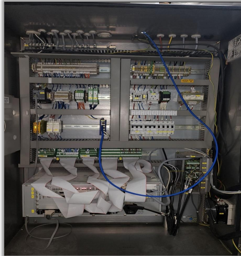
CONTROL PANEL WIRING
